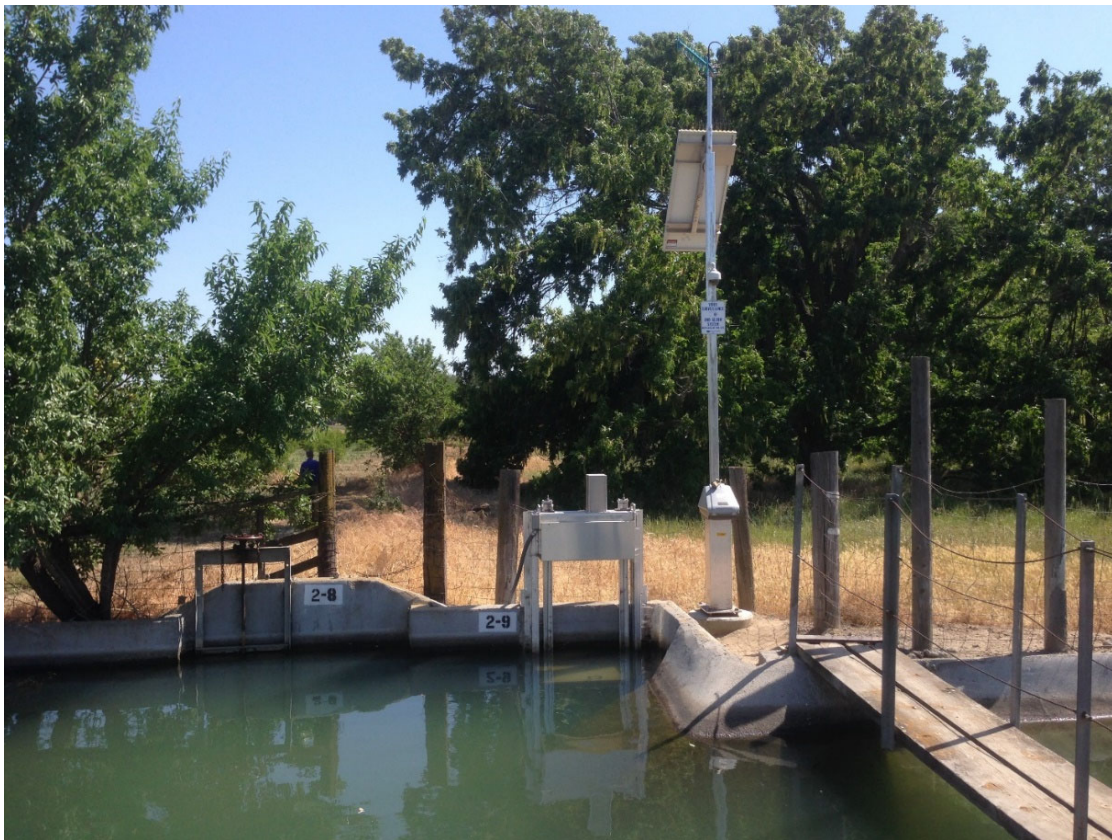
Figure F5.3. Rubicon SlipMeter used for New Permanent Flow Measurement Device; Installed on TID Upper Lateral 3 at Sidegate 2-9. Hach FH950 used to Develop Sidegate-parcel Specific Flow Rate Calibrations for Adjacent Sidegate 2-8.
