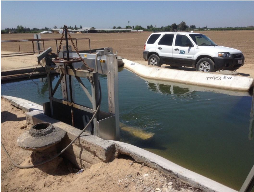
Figure F5.5. Rubicon FlumeMeter used for Sidegate-Parcel Flow Rate Calibrations; Temporarily Installed on TID Upper Lateral 4 at Existing Sidegate 2-4.
