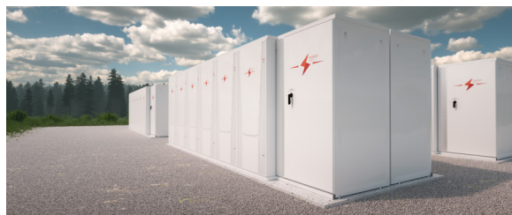
Exploration of battery storage opportunities
