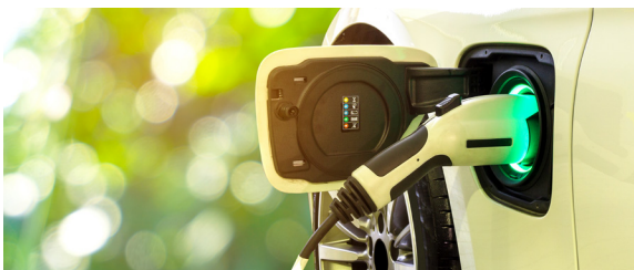
Implementation of TID EV Charging Stations
